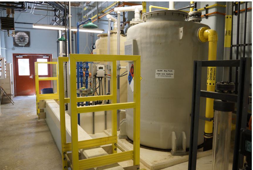
Rockville operations staff at the City’s Water Treatment Plant (top); Water Treatment Plant equipment (bottom)
