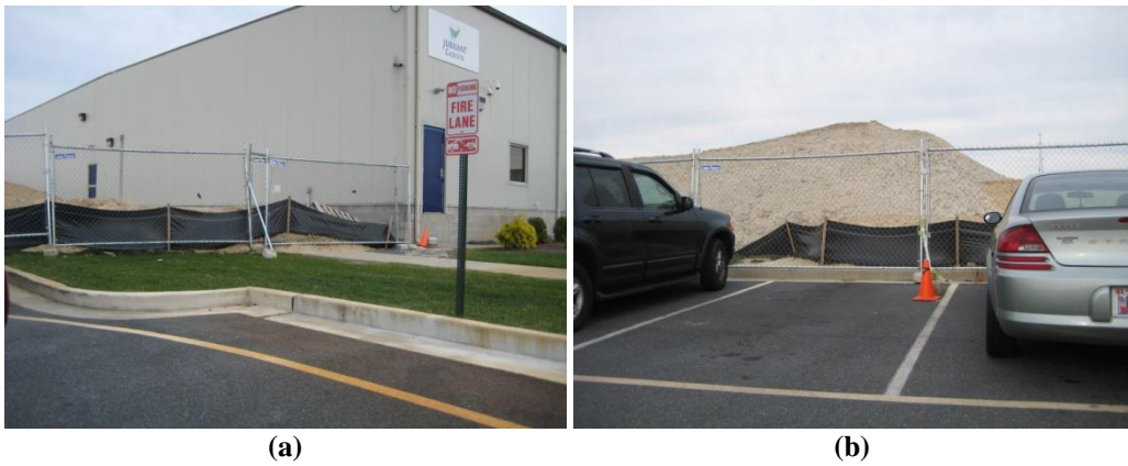
Figure 4.26. HSI_31 (a) and (b) Poor erosion and sediment control (ESC) practices at Jubilant Cadista.
